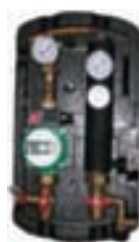
Details of the pump inner with gauges and valves
