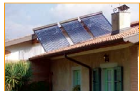
EPL Solar Heating System Installed in Italy, Cagliari (Pitch 42 degree)
